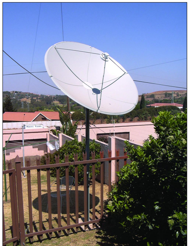
Figure 7 - The 1.8-metre solid dish required to receive C-Band
