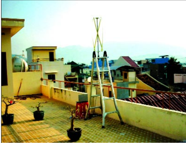
Figure 1 - The antenna mounted on a roof-top ladder
