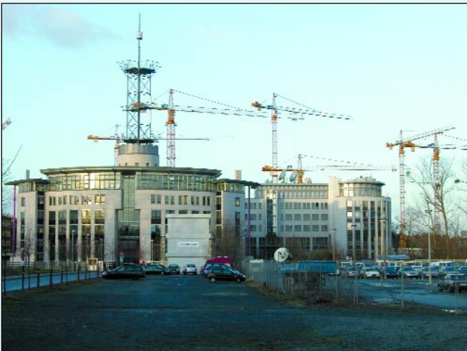
Cranes around EUMETSAT HQ block C-band reception
