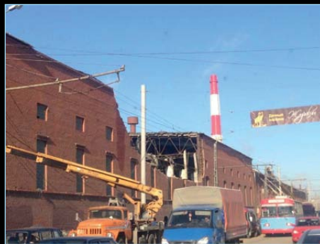
Figure 9 - The Chelyabinsk Zinc Plant with half its roof missing and its wall collapsed. Photo A Pospel / Wikimedia
