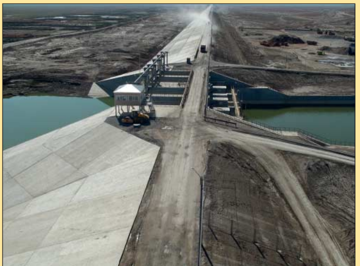
Figure 8 - The Crest of the Koksaray Dam Photo: Kazakhstan Ministry of Emergencies Press Service
