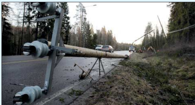
Electrical lines downed by Dagmar
