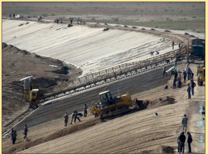
Figure 7 - Construction of the Koksaray Dam in October 2010 Photo: Kazakhstan Ministry of Emergencies Press Service
