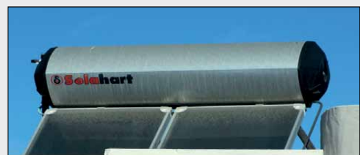
Figure 10 - One of the ubiquitous solar roof-mounted water heating units
