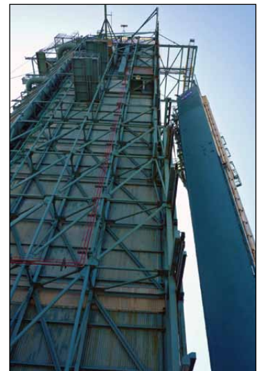
Look up from right to left - fixed umbilical tower and mobile service tower
