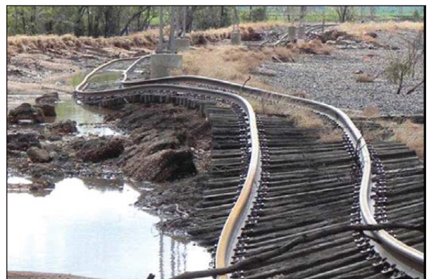
Buckled railway lines
