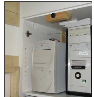
Figure 7 - The Server Room
