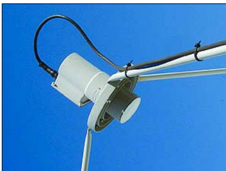
Figure 4 This LNB is slightly off alignment, which may be the reason for a weak signal.
