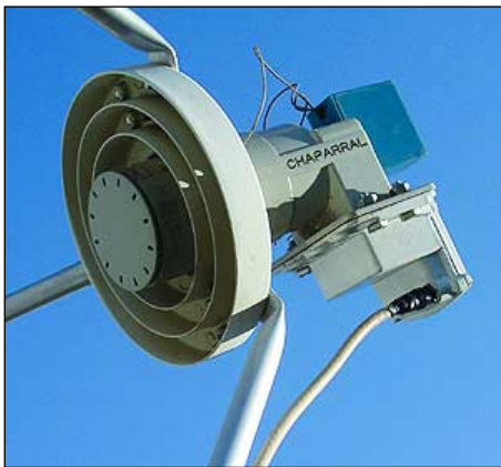
Figure 3 A different view of the finally installed LNB
